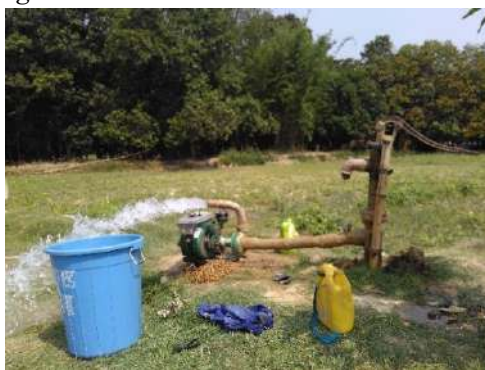
Fig.8 Low head high discharge pump in operation
