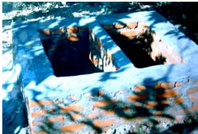
A Two-Tank Unit
