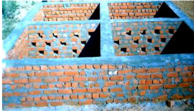
A Four-Tank Unit
