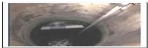
Abandoned Dug Well fitted with Rain Water Harvesting Mechanism
