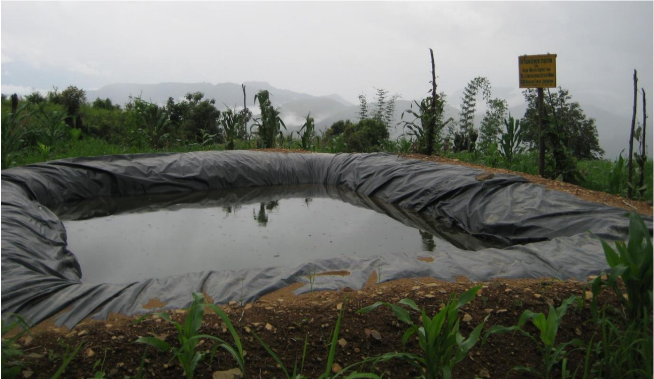
Jalkund having storage capacity of 30,000 litres of water constructed at Longsachung village, Nagaland
