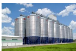
Fig 3: Grain Silos with Aeration System
